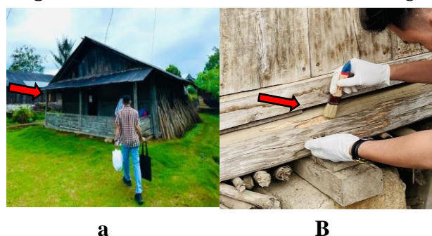
Figure 3. Termite Attack on Building Structures
