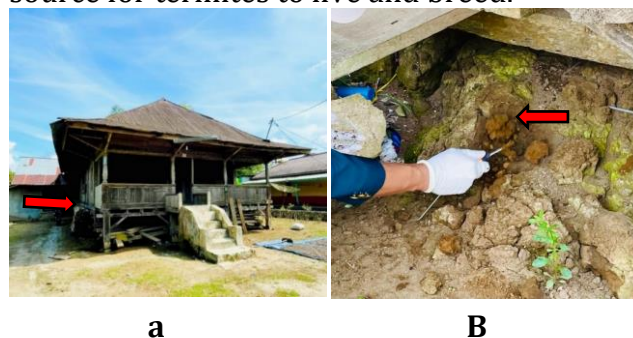
Figure 2. Termite Attack on 85-Year-Old Building
