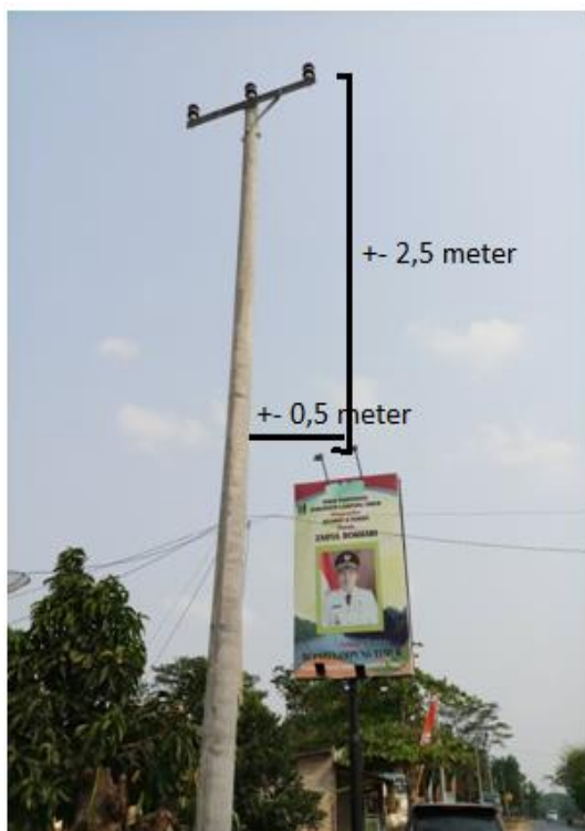
Figure 3. The distance between conductors and billboards.
