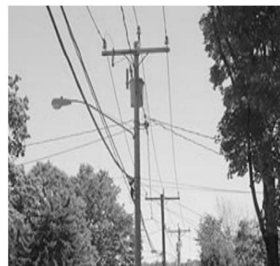
Figure 1. Medium Voltage Air Lines (SUTM)
